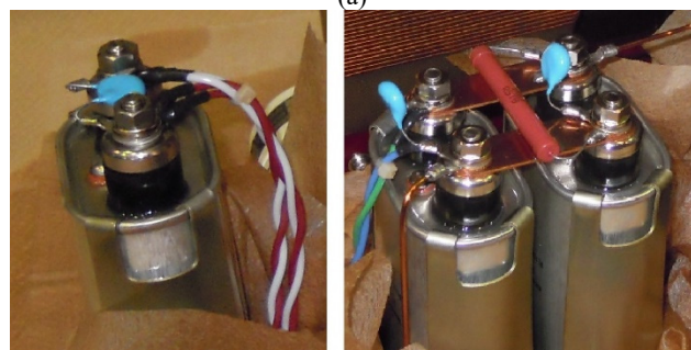
Figure 3: Capacitors that need to be exchanged in pulse transformer tanks. (a) Schematic diagram of pulse transformer tank. Three applicable capacitors are surrounded by red circles. (b) Photos of three capacitor.
