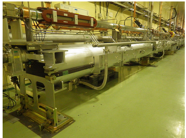
Figure 1: Standard accelerator girder at LINAC.
