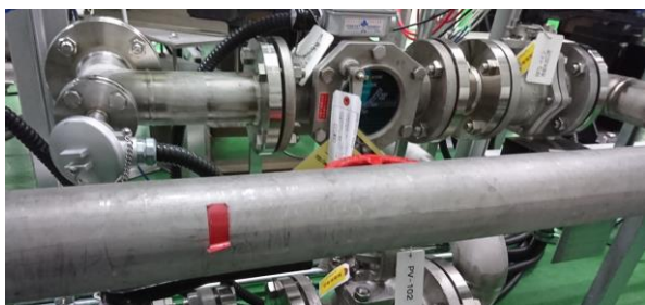
Figure 4: Enlarging RFQ cooling-water pipe diameter to increase flow rate, before (top) and after (bottom) the refurbishment.
