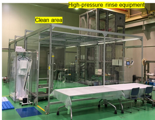
Figure 2: High-pressure rinse facility.
