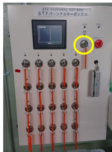
Figure 4: STF tunnel personal key box.
