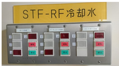
Figure 2: Cooling water operation switch.
