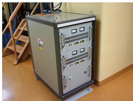
Figure 5: Picture of the newly installed 1 kW transistor amplifier for the cyclotron RF system.
