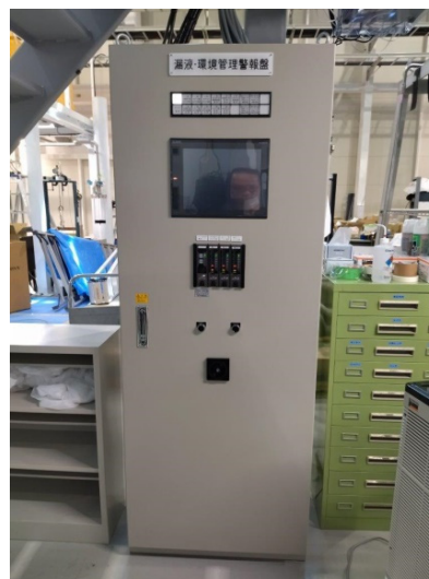
Figure 7: Environmental safety alarm panel to control each safety device.
