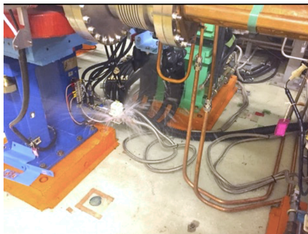
Figure 2: Water leakage from a flow switch.
