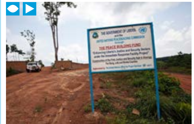
In Gbarnga, construction is underway for a new $3.7 million justice and peace hub, paid for by the UN Peacebuilding Fund and being built by the United Nations Office for Project Services. The facilities will include courts, offices, barracks and training centres for security agencies, and serves much of central Liberia. A sign at the entrance of the Gbarnga Justice and Peace Hub. 13 APRIL 2012/UN PHOTO/STATON WINTER
